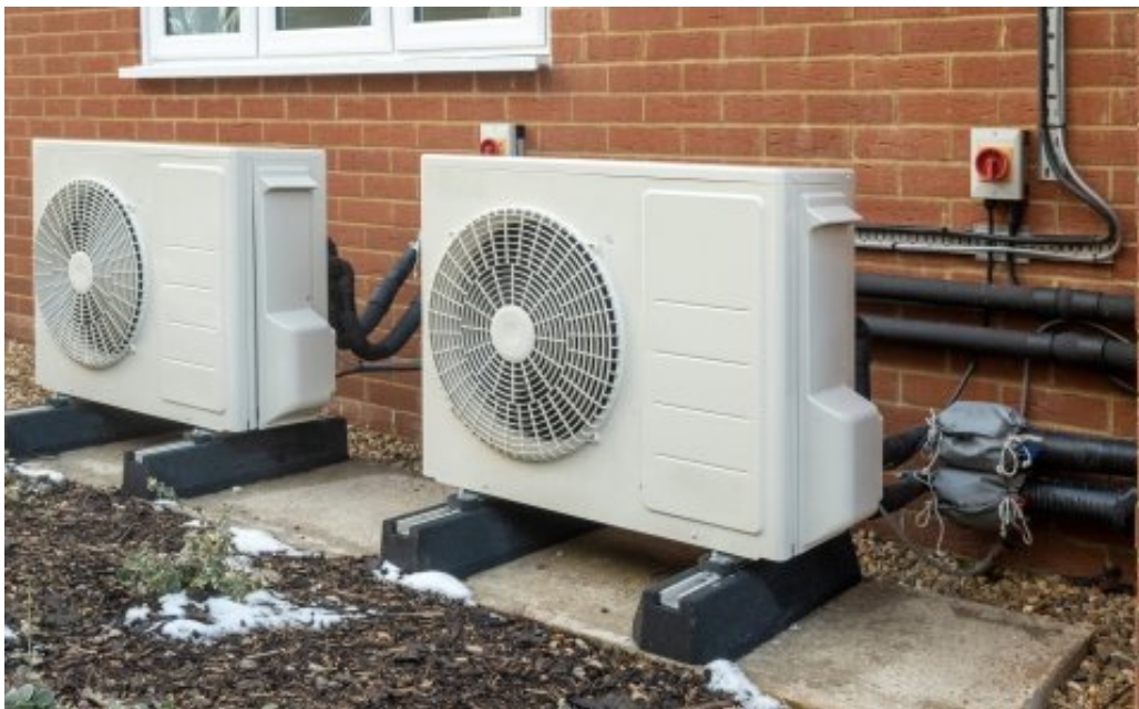
Figure 5.5: Heat Pump outside a building (“Heat Pump System”)
